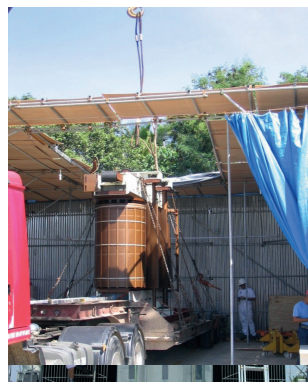
230kV / 50MVAr Reactor
